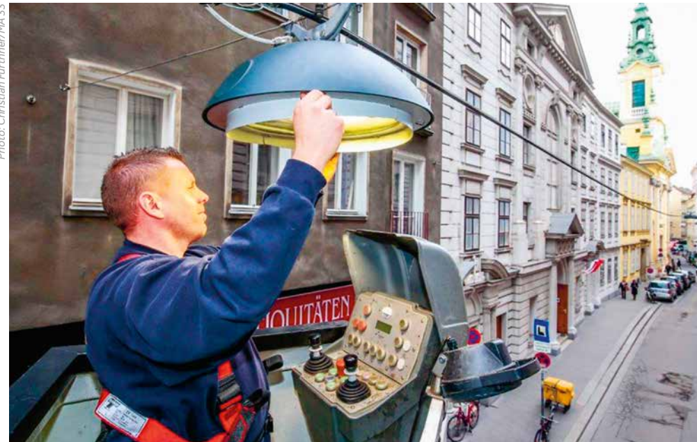
Fig. 3 Switching to LED technology
