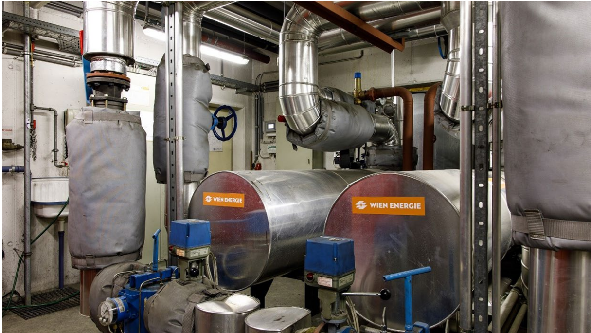
Figure 33: Wien Energie local district heating substation © Wien Energie/Max Kropitz
