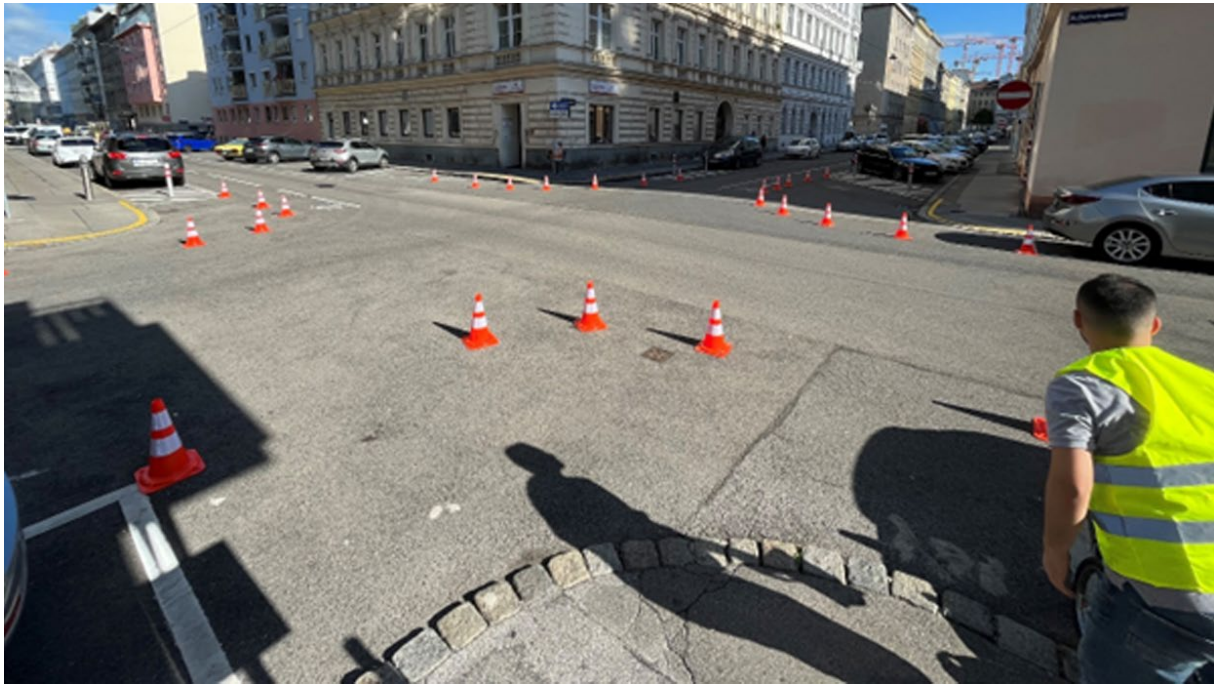
Figure 55: Pop-up pavement extensions: more space for pedestrian safety. © Ulrich Leth
